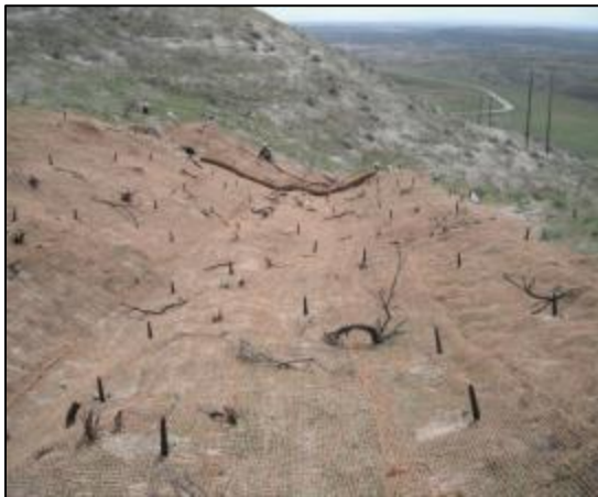
Erosion control matting in place along with wattles and sagebrush seedlings, April 2011
